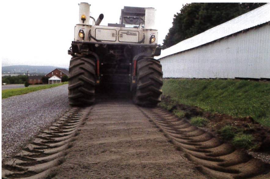
When East Earl Township, Lancaster County, replaced a culvert a few years ago (top), it also elevated the road to keep it from flooding. The township spread stone on the road, and then a reclaiming machine ground up the surface and stone together (above). More stone was added to increase the height, and then new blacktop was applied. (Photos courtesy of East Earl Township.)
